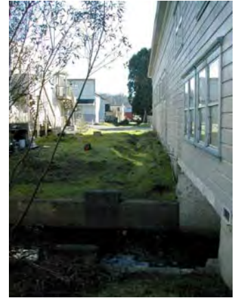
One small trestle over Powers Creek was destroyed in late 1997 and will need to be replaced..
