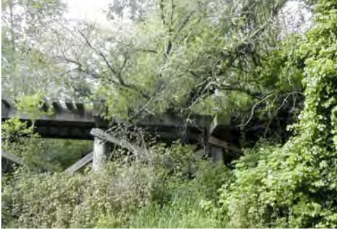
In less than five years since rail and tie were removed, much of the corridor is grown over, and several trees have fallen across trestles.
