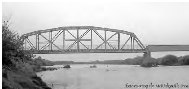
The Hammond Trail Mad River Bridge is just downstream, close to the beach, and of similar steel truss construction – and is substantially more corroded than the A&M bridge.
