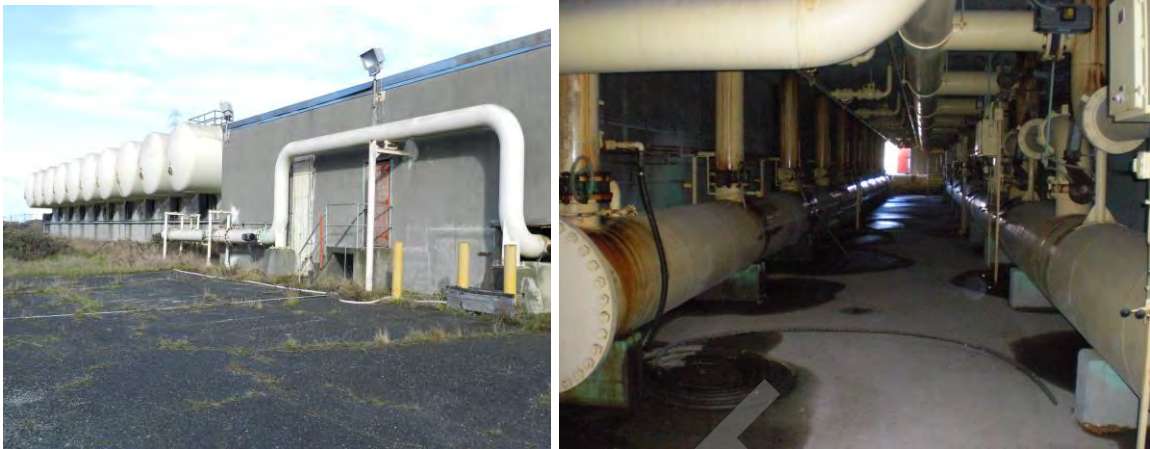
Figure 11 – Photographs of 30MGD Water Treatment Facility
