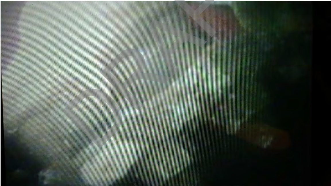
Figure 8 Flange deterioration (previous inspection)
