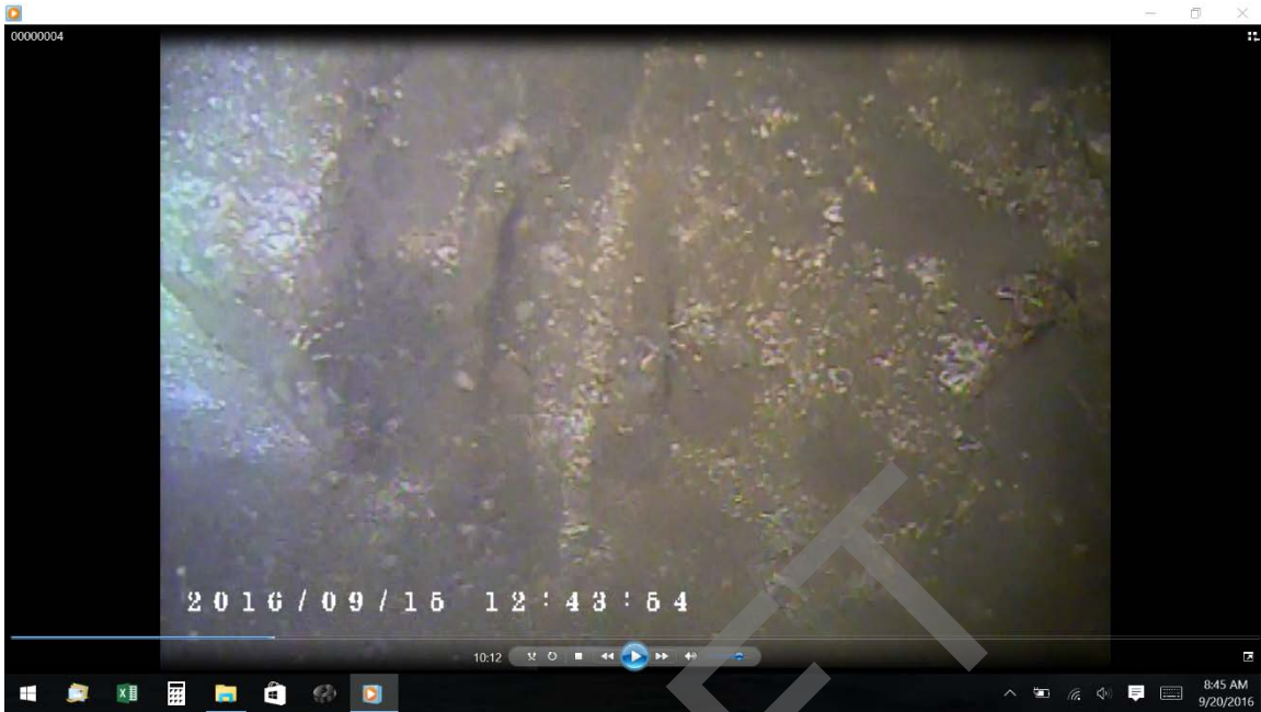
Figure 1 Exposed rebar in external concrete coating.
