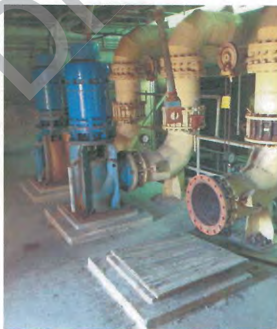
Figure 4. Missing vertical turbine pump in the influent water treatment plant.
