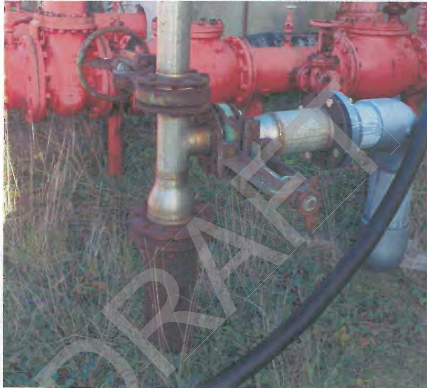
Figure 2. Domestic water 6-inch diameter source pipe on the Freshwater Tissue Pulp Mill site.
