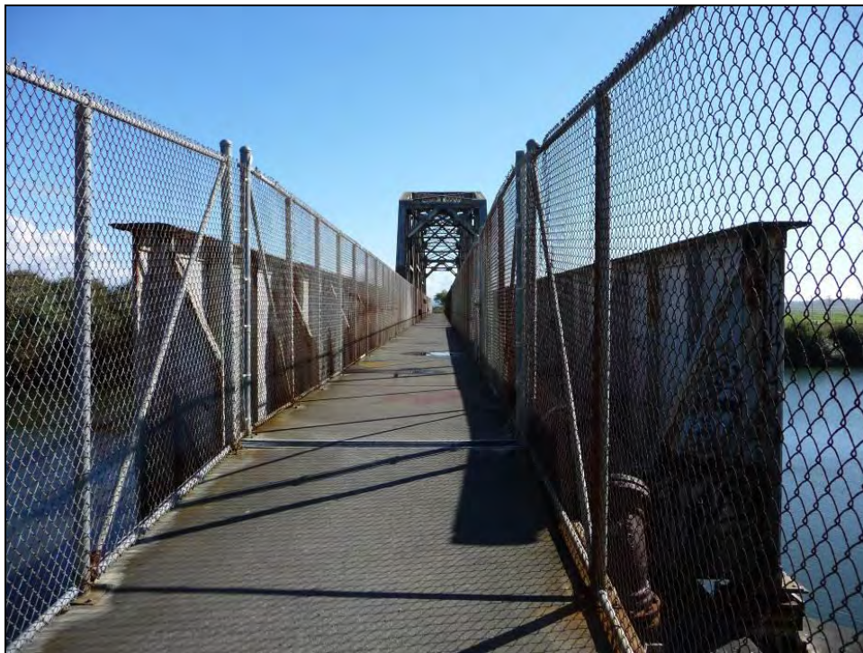
Photograph 2. Span 3 showing deck and sewage line at right, camera facing south, September 25, 2013.
