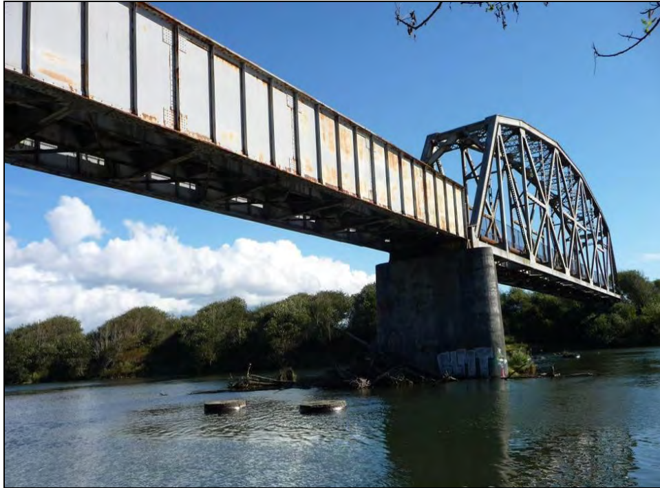
Photograph 1. Two main spans of the Hammond Bridge. Note the two piles just above the water surface from the original bridge, camera facing southeast, September 25, 2013.
